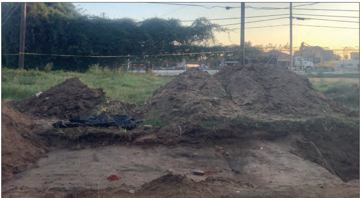
B. View North of Utility Lines in the Central Section of Stripped Area A
