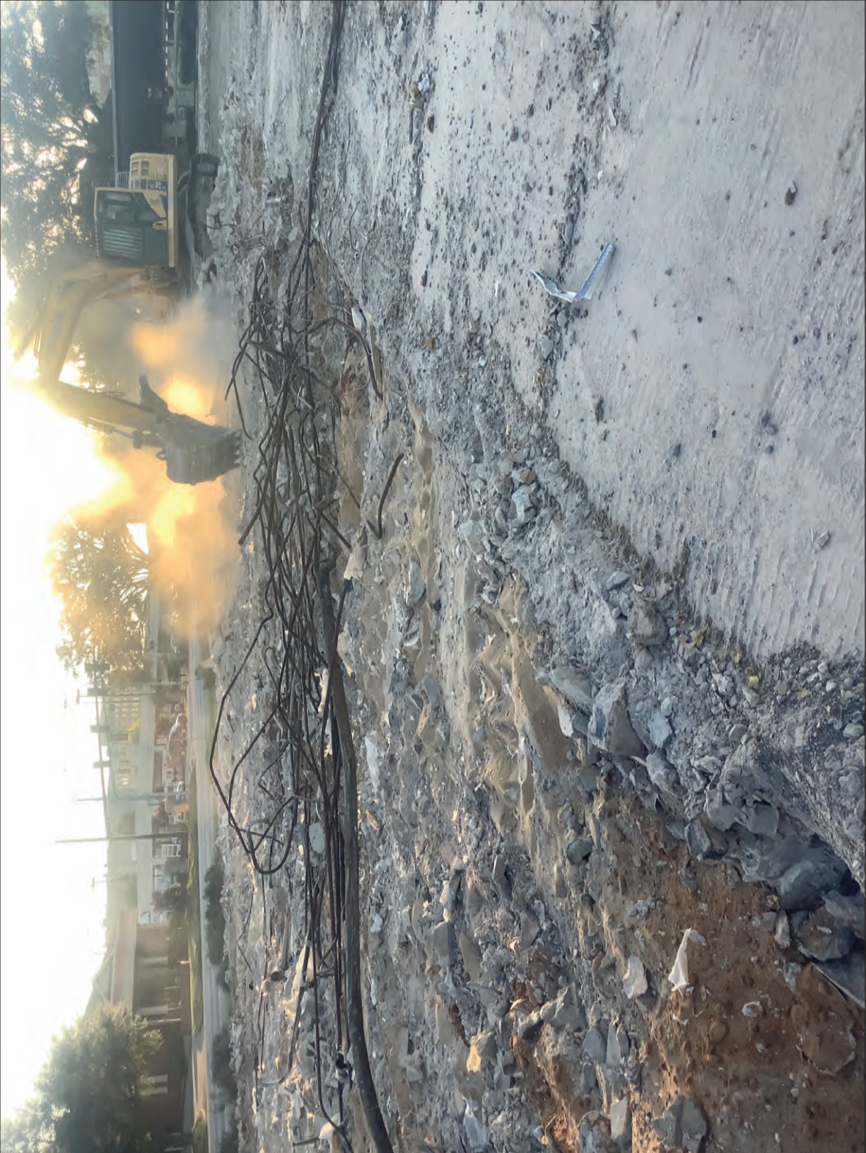
Figure 5.77 Foundation Slab Removal at the Greyhound Bus Station Showing Sandy Fill Soils
